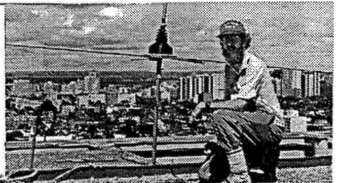
A member of the work crew, Mike Kelly, VE3FFK, getting ready to tune the antenna.
